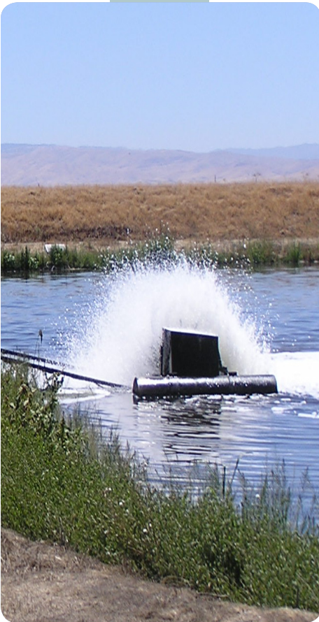
An aeration pond at the Discovery Bay Community Services District wastewater treatment facility. Equipment and process improvements will save a projected $80,000 annually in energy costs, funded by the California Process Optimization Program.
