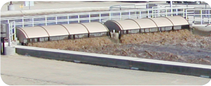
Oxidation ditches at this Discovery Bay CSD facility were retrofitted with sensors and automated controls to reduce energy usage.
